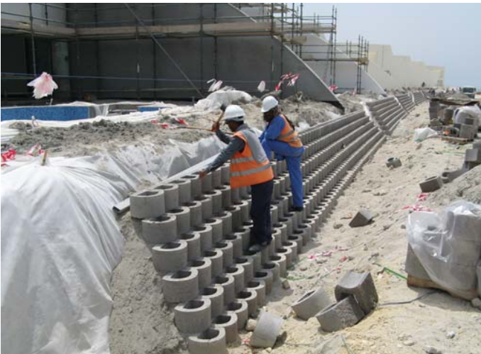
Line 6 in the foreground and line 7 in the background being levelled out.
