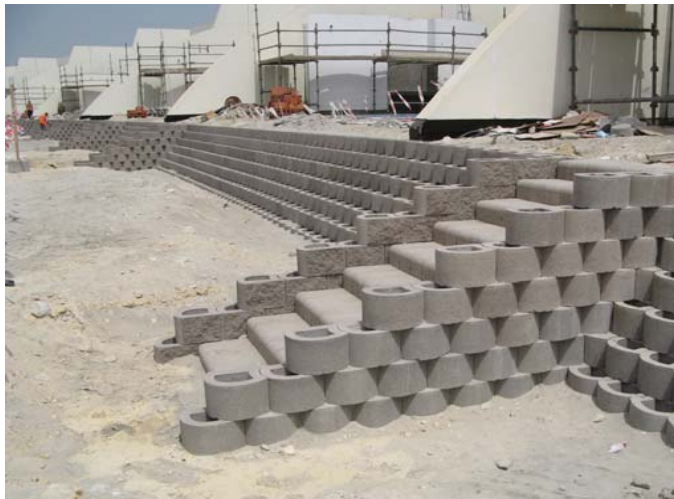
Series of stairways installed with Terraforce 4x4 step blocks and L16 wing walls.
