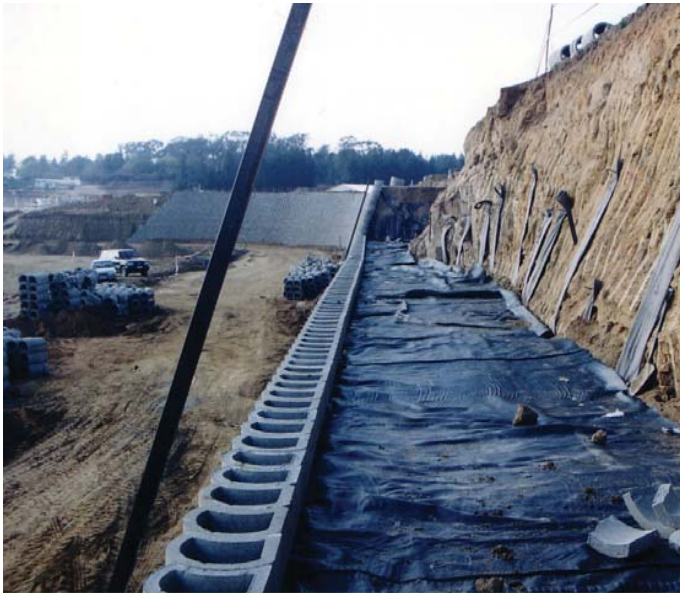
Blocks placed on 25m.p.a. concrete foundation & built to full height in chainages of +/- 60m.
