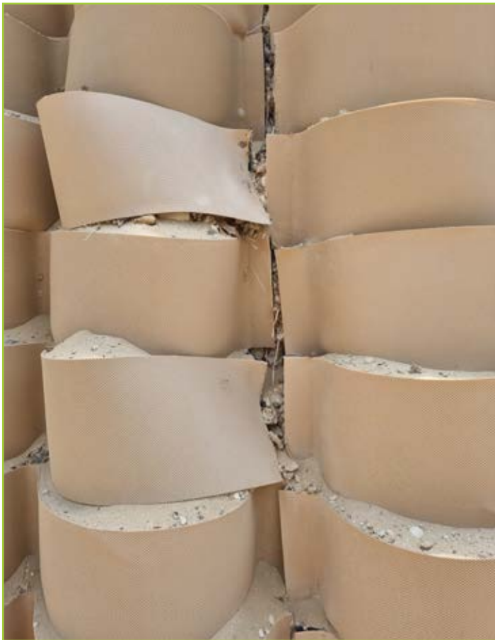
Plastic cell retaining wall degrading in the extreme heat in Dubai
